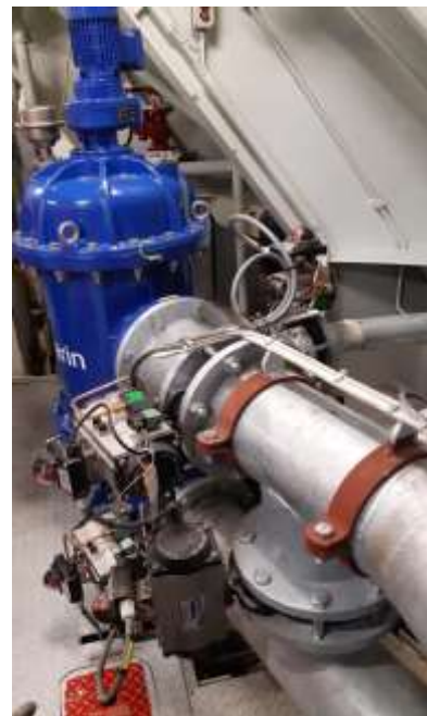
Figure 10: Filter with pneumatic valves.
