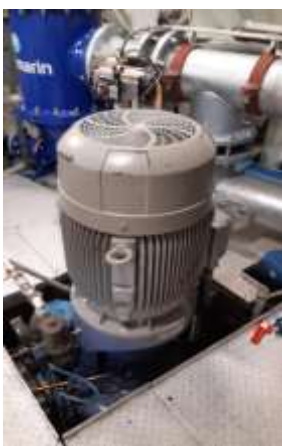
Figure 11: Ballast Water Pump
