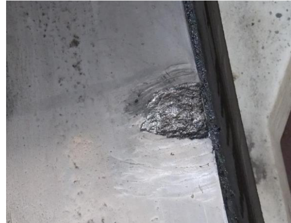
Figure 2 Damage of the ring
