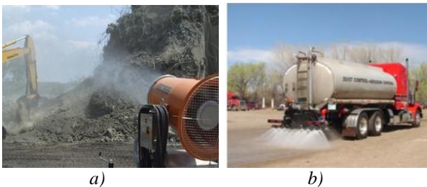
Figure 6: Dust control measure on site a) water spray; b) water tanker with spray.
