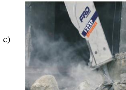
Figure 1: Air pollution during work activities with technological equipments a) drilling machine; b) crusher; c) hydraulic hammer for demolition.
